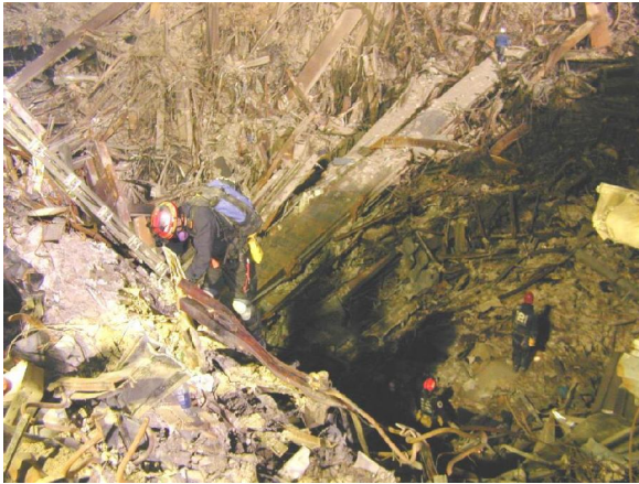
Figure 3-1 - GZ workers descend into the subbasements below WTC2. While there is extensive damage, there is little building debris at the bottom of the hole. There is no sign of molten metal. A worker in the distance walks along a massive core column.
