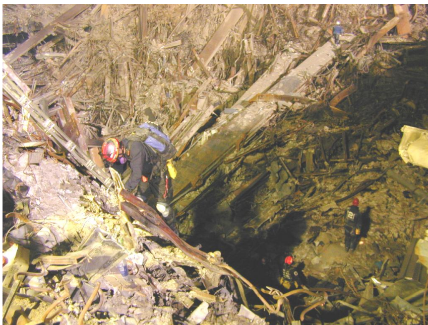
Figure 3-1 - GZ workers descend into the subbasements below WTC2. While there is extensive damage, there is little building debris at the bottom of the hole. There is no sign of molten metal. A worker in the distance walks along a massive core column.
