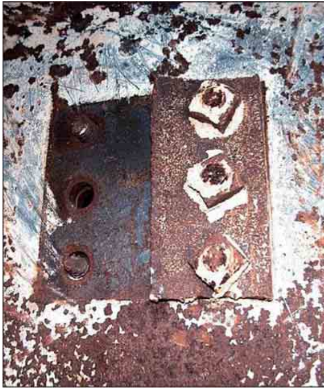
Figure 71. Figure 6-8, Failed shear connection of beam web to column web. Page 8 of 16 of pdf (labeled page 6-8 of FEMA report), http://www.fema.gov/pdf/library/fema403_ch6.pdf fema403_ch608p8a.jpg
