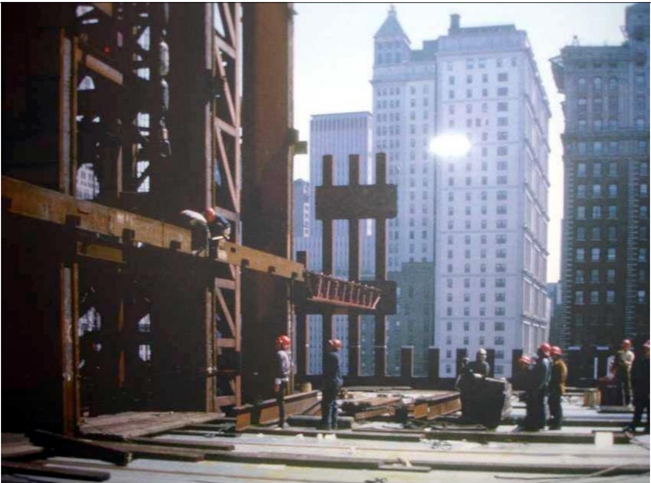
Figure 1. The massive core columns of the WTC, as seen during construction, Because of their mass, they would be an enormous heat sink.
